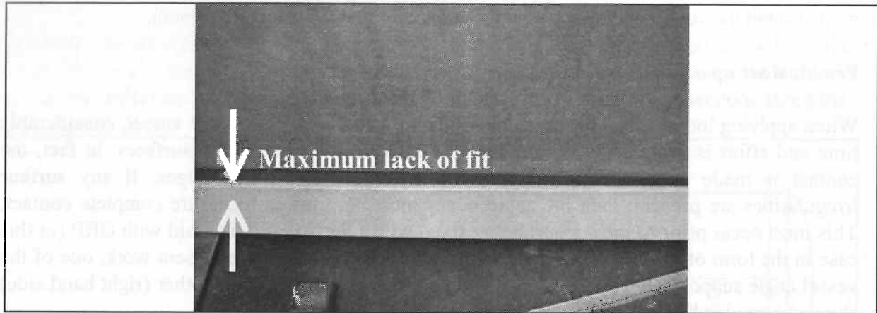
Fig. 8 Lack of fit between shell and angle section
